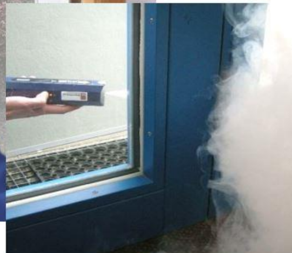
Visualization of leakages with fog
